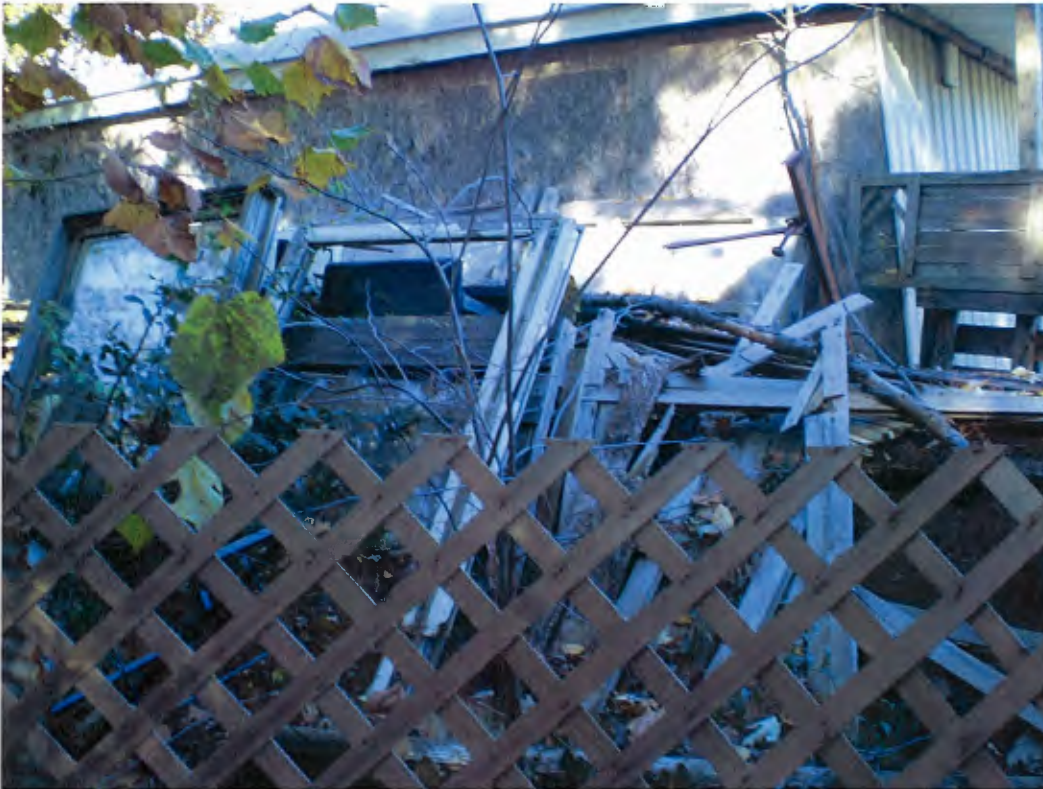
Date: 11-15-07 Time: 10:09am Direction: N Photo by: P. Fatka Exposure #: 005 Comments: GC/DD in the area south of the building.
